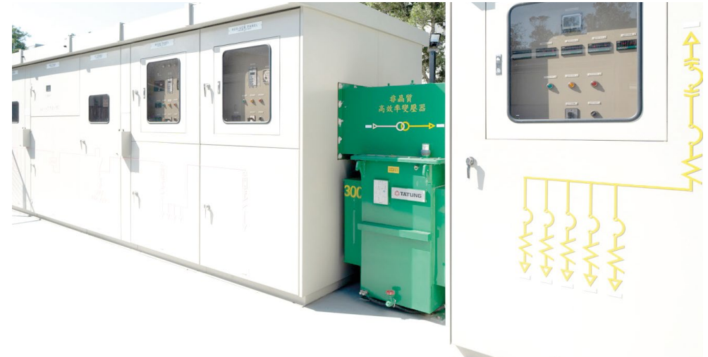
The first E-dReg energy storage system (6MW) in Taiwan
