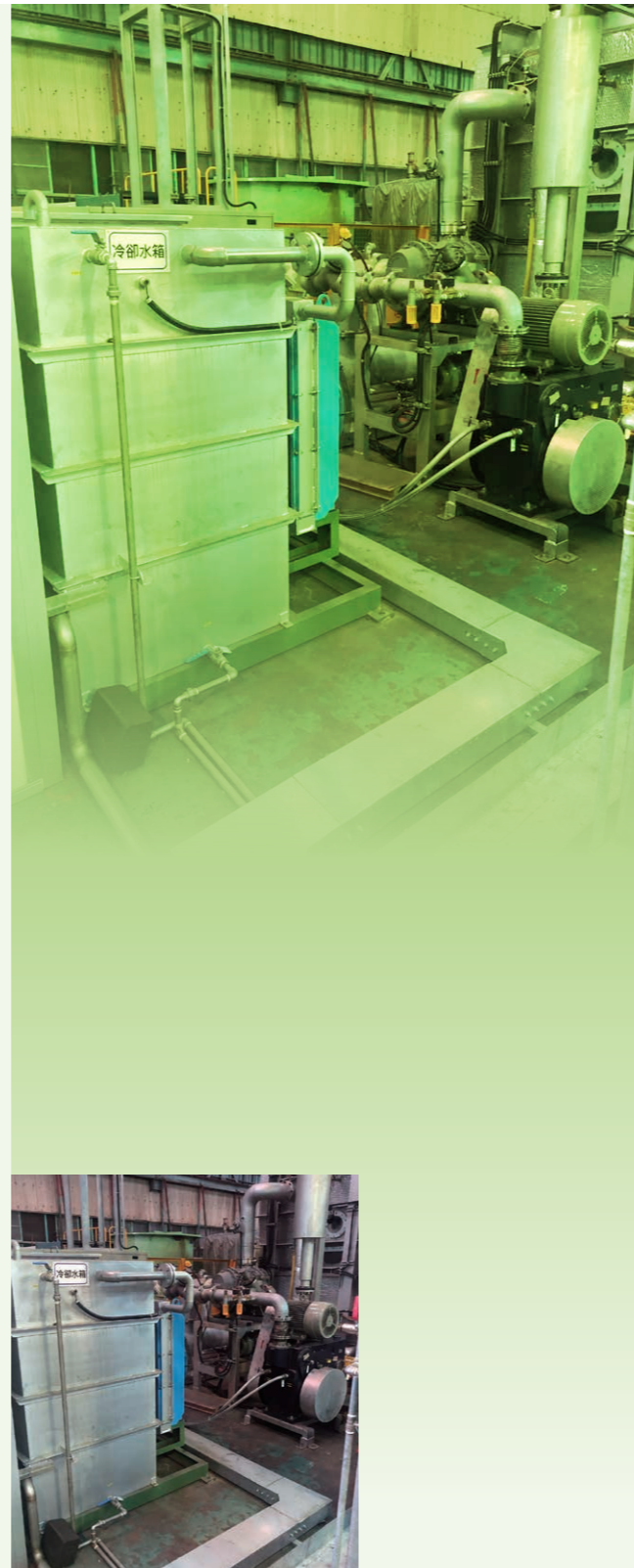
New installed cooling water circulation system for transformer drier in Tayuan Plant
