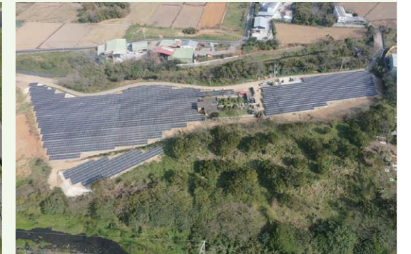
PV solar system at No. 4 cemetery, Xinwu District, Taoyuan City
